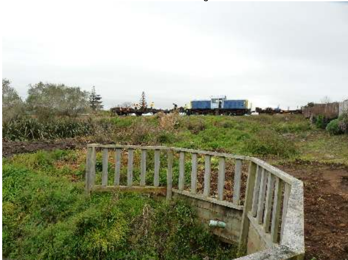
Adding fill behind the retaining walls at Nelson St. Photo D. Bettridge.
