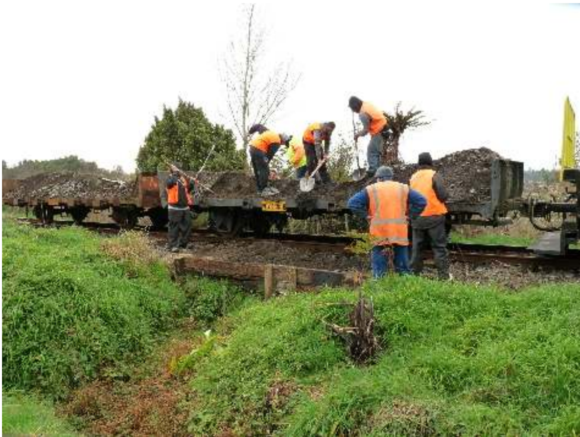
Back filling the swamp drainage culvert retaining wall at Kohatu. Photo D.Bettridge
